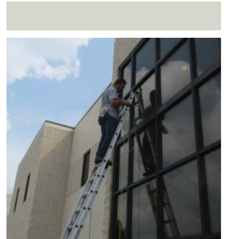
After 25 years of howling winds, melting sunshine, freezing, thawing, battering rains, and even a couple of earth tremors, the windows on the front of the Convention's building needed some repair. Rain was leaking around some of the window joints into the foyer.
